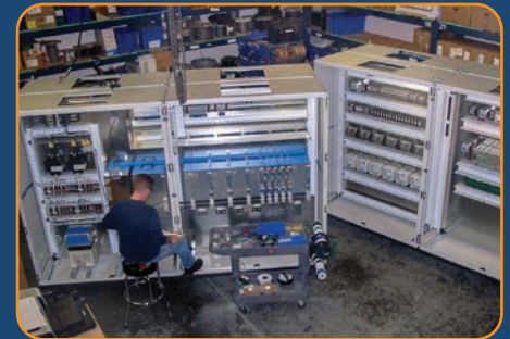
Janicki UL Cabinet Shop
